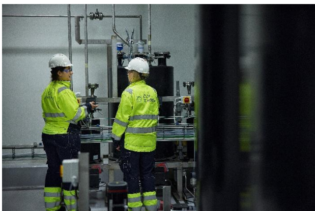
Completed: Commissioning of AlphaOne completed
