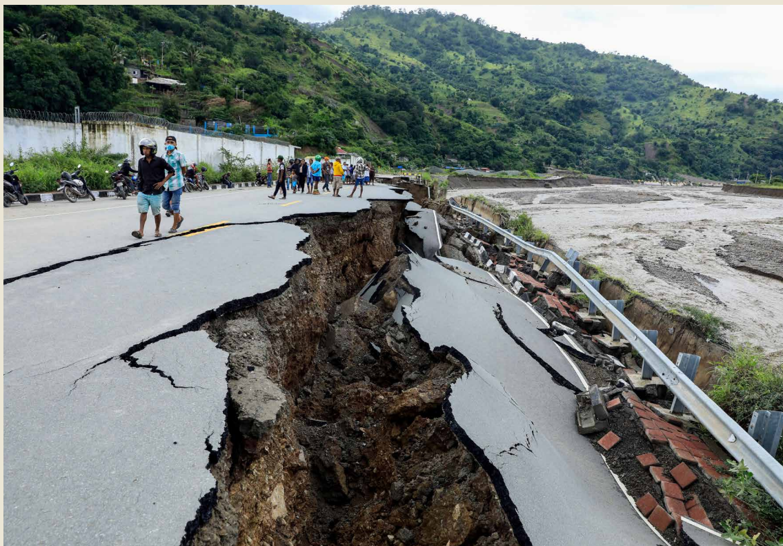
A damaged road in the aftermath of floods in Dili, East Timor, April 2021. Scores were killed and dozens went missing as floods and landslides caused by torrential rains hit the eastern part of Indonesia and East Timor. Photo: Antonio Dasiparu/EPA-EFE/Shutterstock
